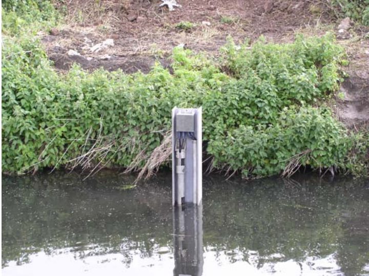
Photo 3: Close-up of installed column/sensor mounting, column flange protects probe from debris
