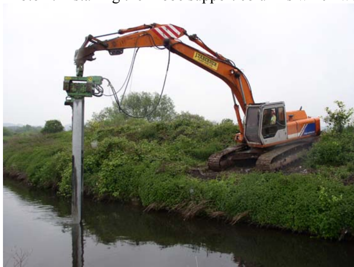
Photo 2: Installing the Probe support columns which were piled approx 2.5 meters into river bed
