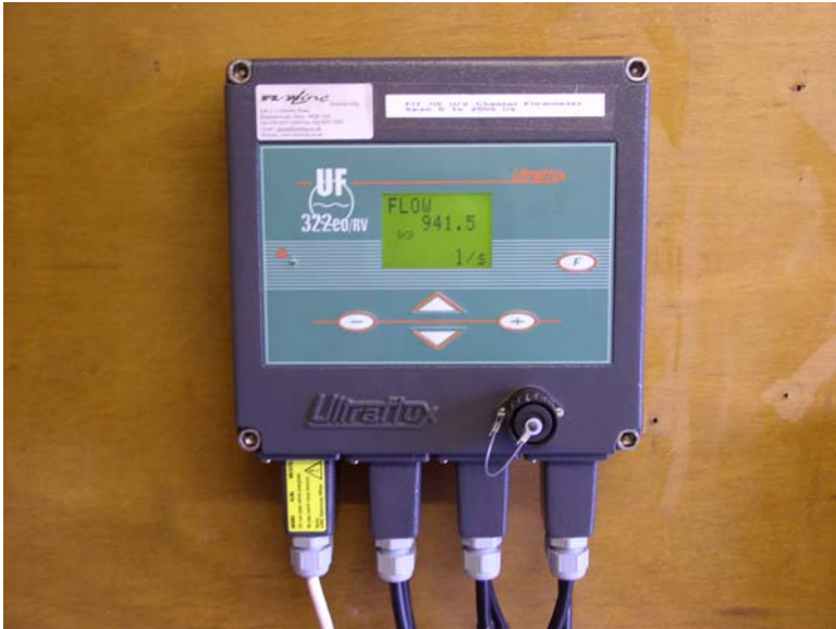
Photo 4: Close up of control unit.
