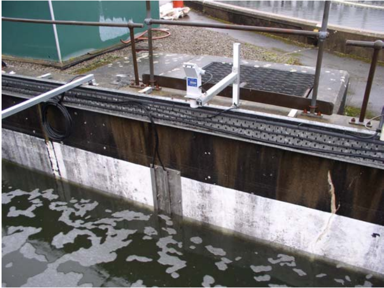
Photo 3: Close-up of installed sensor mounting at normal operating level, Ultrasonic Level sensor is shown above channel
