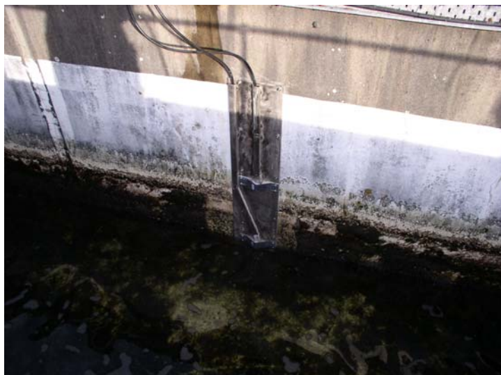
Photo 2: One probe support plate showing high and low level probes. Note St.St protection covers for cables
